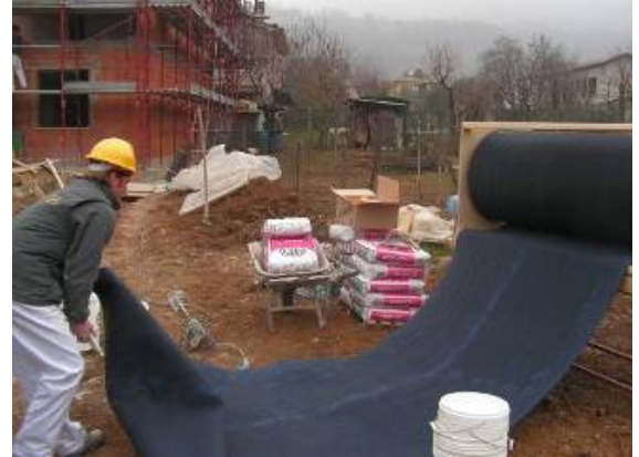
Precut lengths in staging area for ease of handling. Cuts with scissors or utility knife
