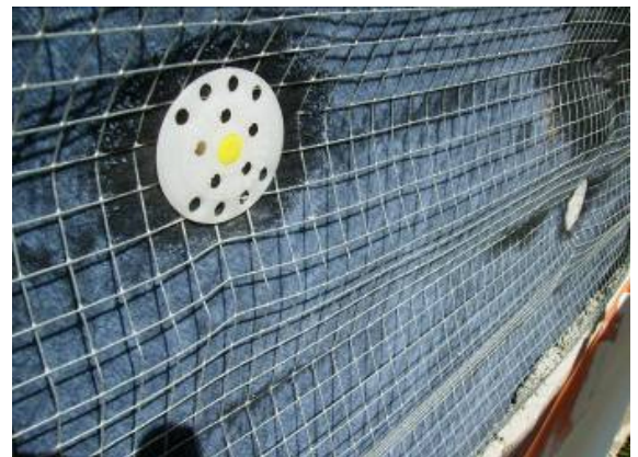
Use appropriate substrate fasteners or construction adhesive. Install final wall finish directly on top
